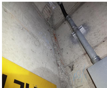
Sta.400~420m Type ④ 균열 0.3/1.0
