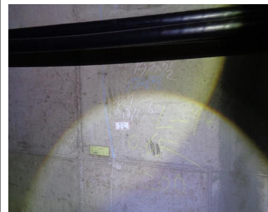
Sta.1880~1900m Type ② 균열 0.3/2.6
