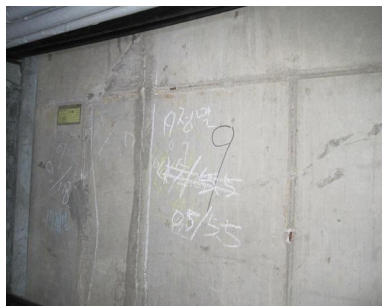
Sta.180~200m Type ② 균열 0.5/5.5
