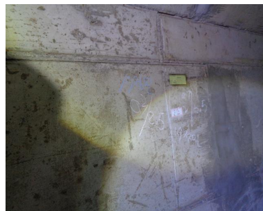
Sta.1760~1780m Type ② 균열 0.3/2.5
